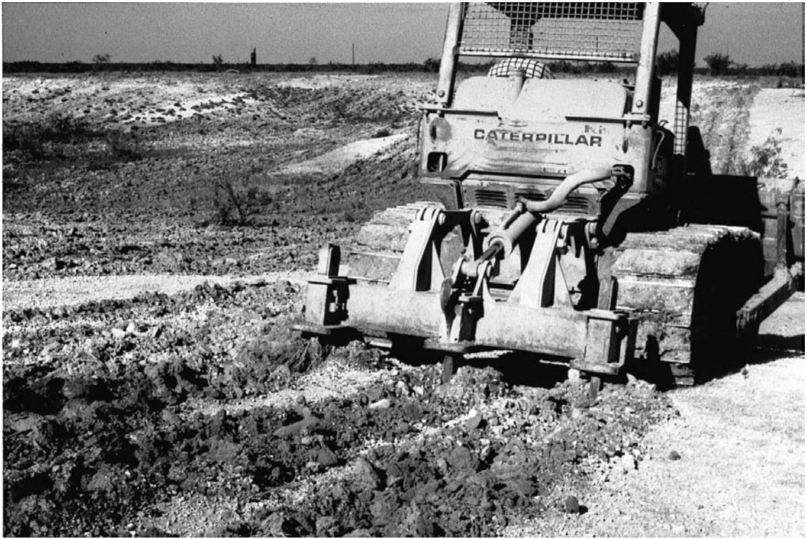
Fig. 6.9. Deep ripping (0.4–0.6 m) this highly compacted substrate in west Texas was necessary before water would move into the soil. Ripping or deep ploughing was necessary to get any establishment of planted species in this seedbed.
