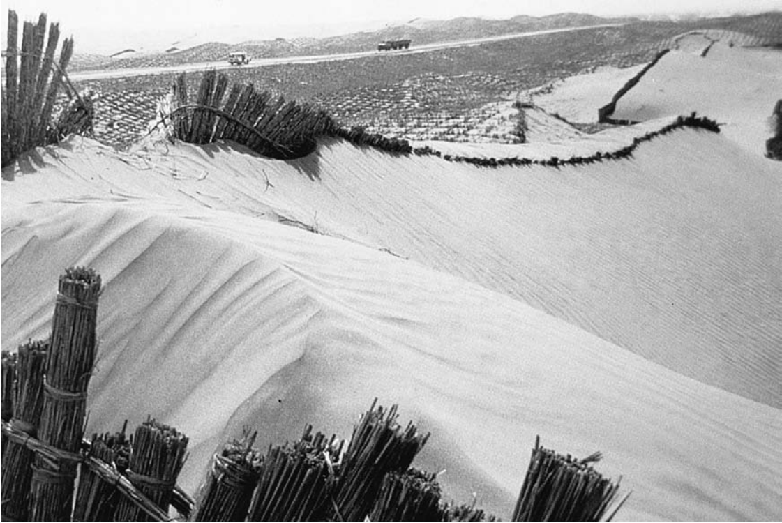
Fig. 6.8. Aboveground obstacles used to reduce sand deposition on the highway through the Taklimakan Desert in western China. The sand fence and the 1 m squares were created from crop stubble and hand thatched into the sand. These structures are often used as a temporary measure to facilitate the establishment of seeded species. However, here they are maintained permanently, because no vegetation grows in this portion of the Taklimakan Desert.
