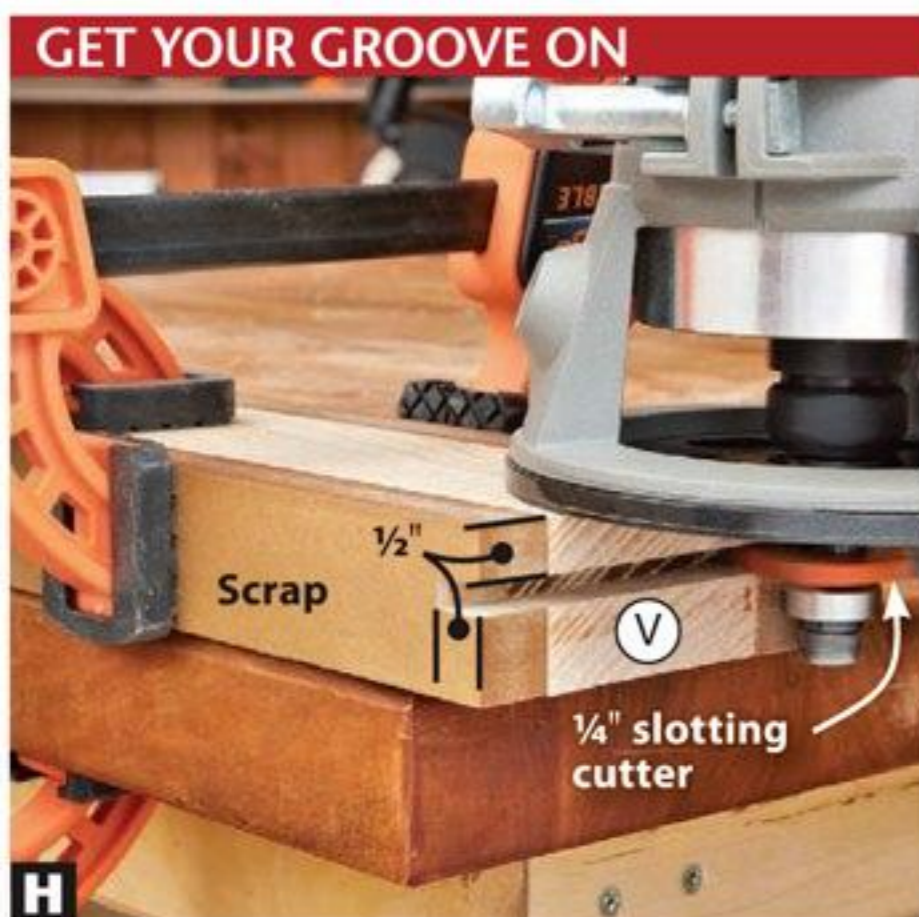
H Rout a groove \frac{1}{2} " from one face, flip the trim (V) over and rout from the opposite face to create a centered groove.
