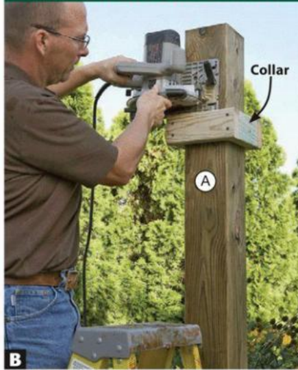
B Screw a collar to the post (A) to guide your circular saw around all four sides of the post. Complete the cut with a handsaw.
