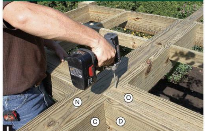
I Secure the loose end of the cross tie (N) with 3" deck screws. Then screw the short cross ties (O) to the crossbeams (C).
