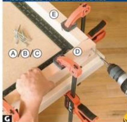
G Clamp the long and short rails (D, E) to the tabletop and check for square. Clamps hold the rails together while you drive 2½" screws.
