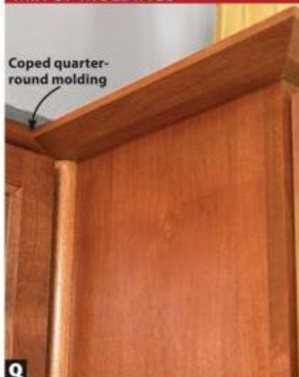
Q Chamfered molding tops the bumped-out cabinets. Flexible quarter-round molding follows the soffit above the cabinets.
