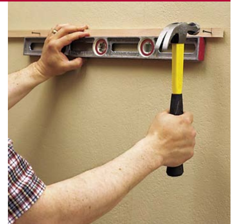
With the spacing strip braced atop a level, it's easy to mark screw and anchor locations with just two taps of a hammer.
