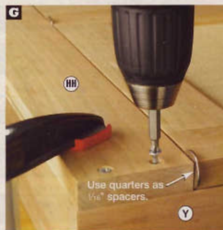
Inserting quarters between the doors and the filler (HH), glue and clamp the filler in place. Drill pilot holes into the sides (Y), and drive the screws.
