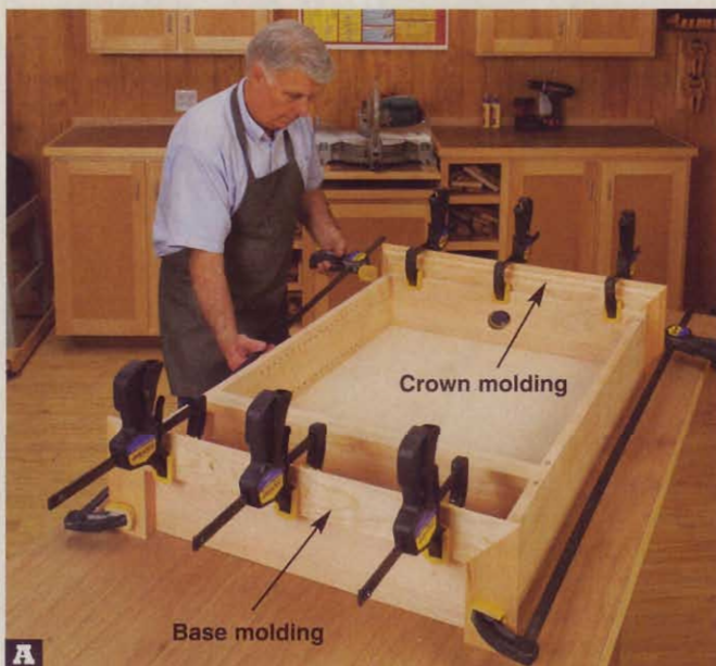
A Glue and clamp the crown molding assembly (G/H/I) and base molding assembly (G/H) to the case, centered side-to-side and flush with the case's back.
