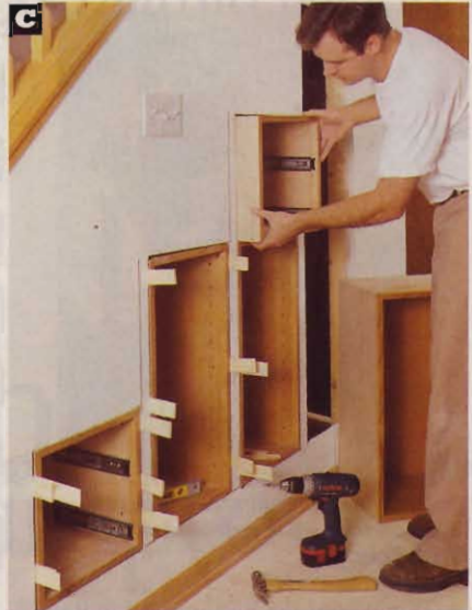
To make the box plumb in its wall opening, insert shims between the box and wall studs.
