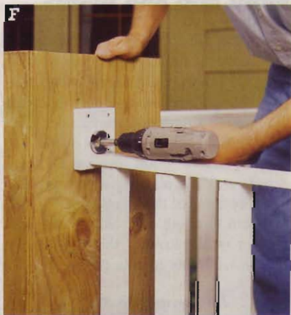
Guided by the hole in the upper bracket, drill a 1\frac{1}{16} " hole through the column. Repeat at the railing's other end.
