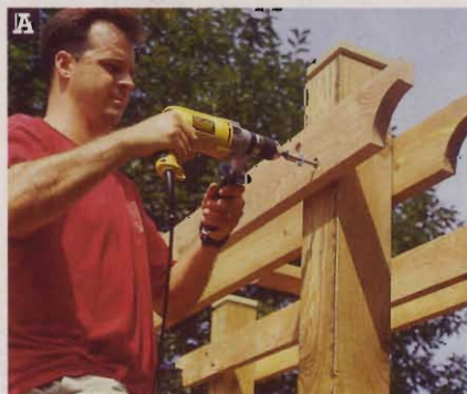
Fasten the main joists to the posts with lag screws and flat washers.
