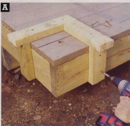
A Fasten the cleats (C, D, E) to the deck with 3"-long deck screws.
