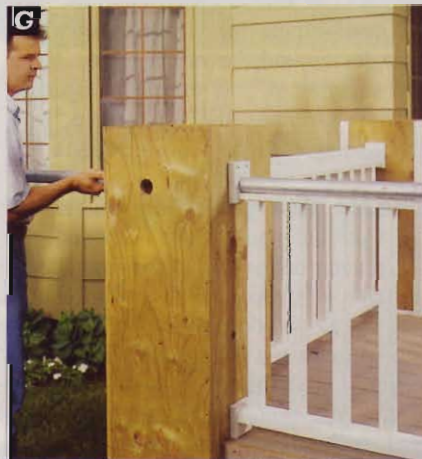
A hole in the column face opposite the railing facilitates the installation of the 1\frac{1}{2} " galvanized steel pipe.
