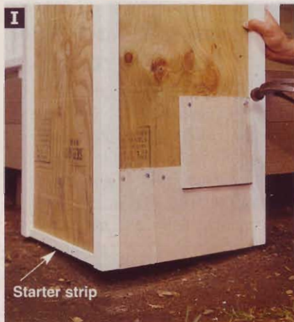
Starter strips nailed to the bottom of each column side give the first course of shingles the appropriate slope.
