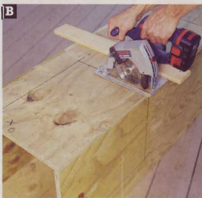
B To guide your saw, temporarily nail a short, straight board to the column.
