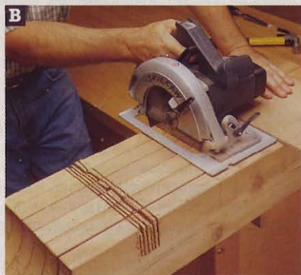
Set your saw to cut 2 1/4" deep. Clamp a straightedge to the joists, and cut a series of kerfs to define the notches.
