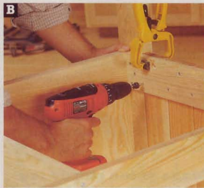
To give the bench a clean appearance, drive the 1 1/4" deck screws into the end boards from inside the carcass.
