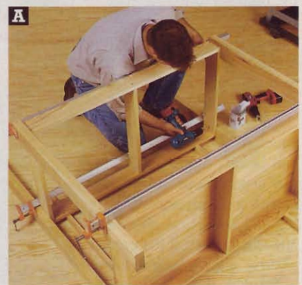
Drill countersunk shank and pilot holes, then drive 2" deck screws through the frame assemblies into the legs.
