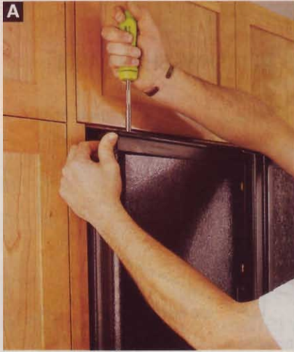
A First, loosen the screws that hold down the plastic panel retainers on the tops of the refrigerator doors.
