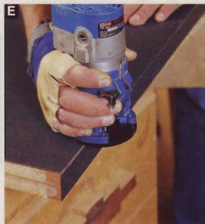
A piloted \frac{1}{2} " flush trimming bit in a handheld router smoothly removes extra laminate from the edge joint.
