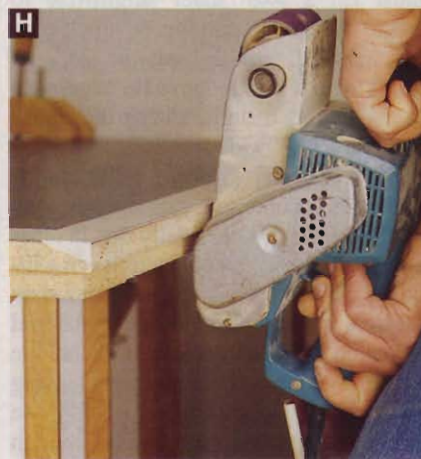
Sanding to the scribe line at a slight angle provides a tighter fit to the wall because the sharp edge cuts into it.
