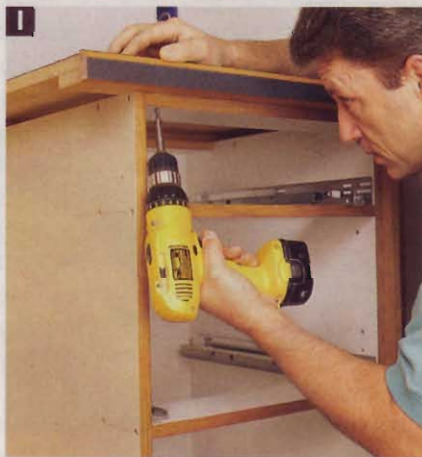
I Fastening the countertop with wood screws through the cabinet spreaders allows later replacement if necessary.
