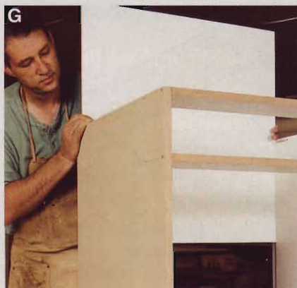
G Slide the back into place without glue. That flexibility will come in handy if you need to adjust the cabinet slightly for squareness during installation.
