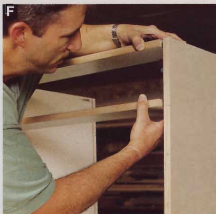
F After you've attached the sides to the bottom, there's still enough "give" to allow the installation of the drawer divider and top front rail.
