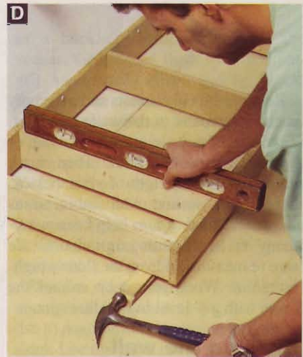
Screw the toekick to the wall, then adjust it horizontally with a level and shims. Later, trim off any protruding ends of the shims with a handsaw.
