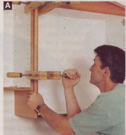
A Use clean, smooth handscrew clamps to align cabinets. You can apply adequate pressure without damaging the wood.
