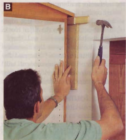
B Protect the wall! with a board when you use shims like this. Remove the shims after screwing the cabinet to the wall.
