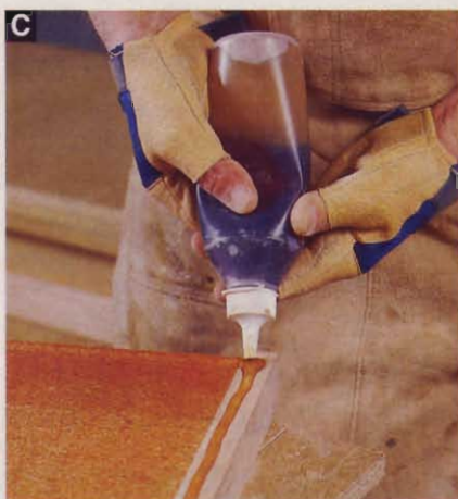
Polyurethane glue on the edging provides a waterproof bond between the wood and the plastic laminate. Apply it after the contact cement dries.
