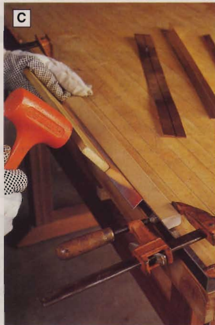
C For straight, even bends, use a long block of wood when forming the copper ridge caps.
