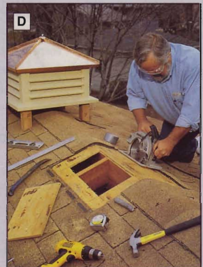
D Mark the cutlines, remove all the nails, and use a circular saw to cut the opening to size.
