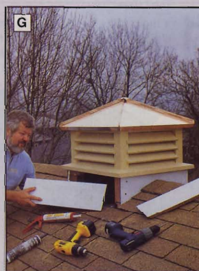
G To prevent moisture from penetrating, the skirting pieces must be cut for a tight fit. Caulk all joints.
