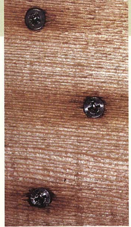
Fasteners open up wood cells that release staining extractives when water soaks the wood.
