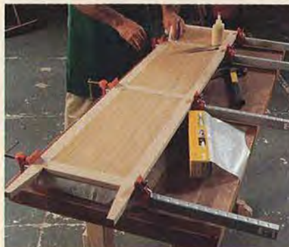
Use plywood spacers when clamping each frame together to help keep the frame members square and aligned.
