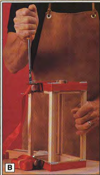
Tighten a pair of band clamps to secure the four frames until the glue dries.
