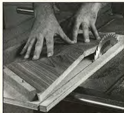
Trim the mating edge of each roof half-section on the table saw.
