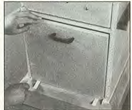
Center the drawer face in the opening, and adhere it to the drawer.
