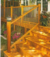
When mounting the stair rails, align the upper ends with the rails on the deck. Then drive screws into the posts to secure the rails.
