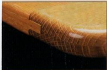
▲ A solid-wood panel will swell during humid months, causing the tongue to extend past the breadboard end.
