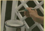
Exterior Latex Paint. After the latticework is nailed in place, I touched up the holes with spackling and exterior latex paint.
