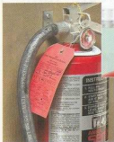
▲ Annual Inspection. A yearly inspection ensures the extinguisher is in good working condition.
