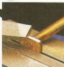
▲ T-Bolts. Lightly file down the sides of the toilet bolts so they slide smoothly in the slots.
