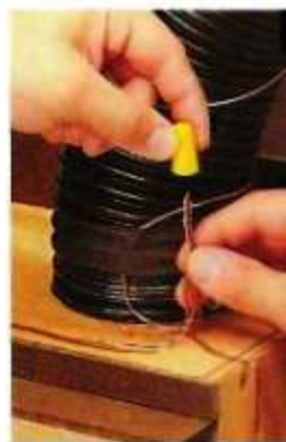
▲ To complete the grounding path, "tie" the ends of the wires together with wire nuts.
