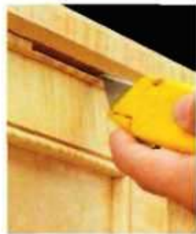
▲ To lay out the location of the hinge on the lid, simply score a line using the mortise in the chest as a guide.
