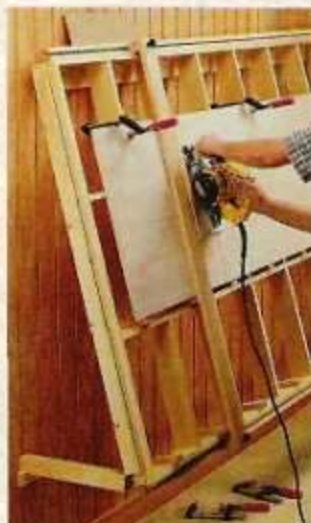
C. Partial Sheets. A row of support blocks holds partial sheets at a convenient height.
