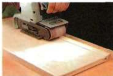
Edging. Sanding wood edging flush with a plywood surface showed how much control the sanders provided.
