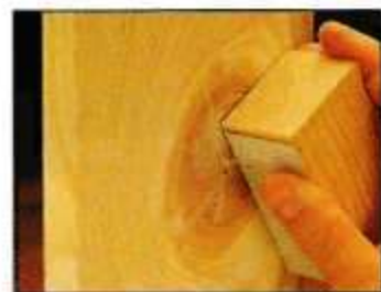
filling all the holes and gaps, allow it to dry overnight before sanding and finishing.
