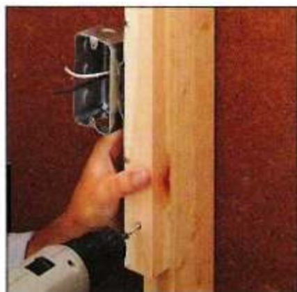
Step 1. Before you begin work on the ceiling or walls, you'll need to extend all of your electrical boxes.
