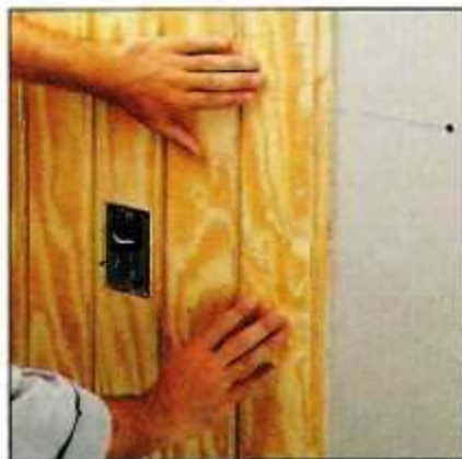
Step 5. A second layer (either drywall or T1-11) will help further increase the STC of the wall and block noise.
