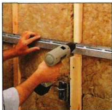
Step 3. With the sound blanket in place, screw lengths of resilient channel to the studs or joists.
