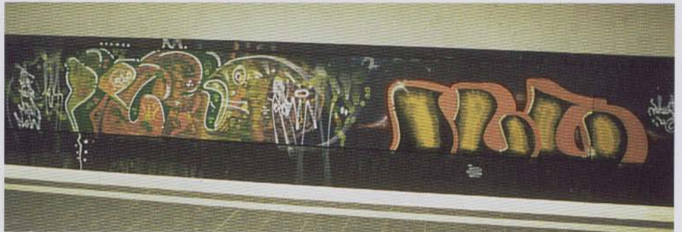
Ilcs, Ilc on line 13. The line was built in the 60's and the walls are raw concrete.
